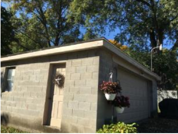
second garage no gutters
