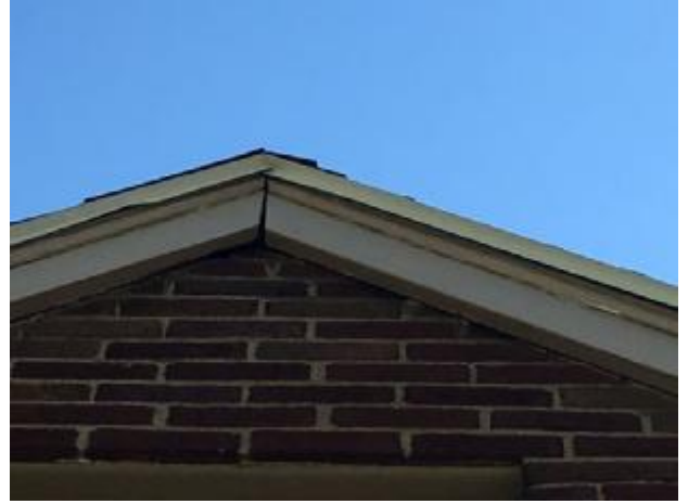
Fascia needs caulked
