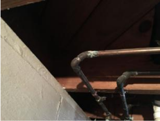
Hot water tank hot line leaking
