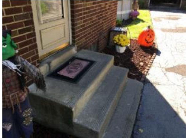
Side porch hand rails needed
