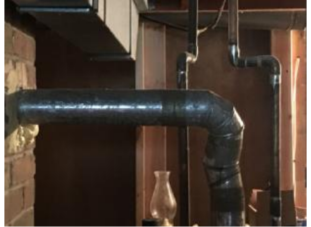
Hot water tank venting
