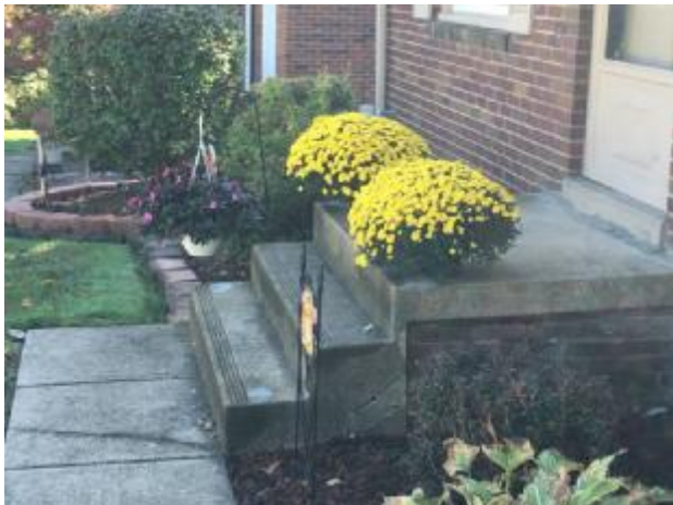
Front porch needs hand rails
