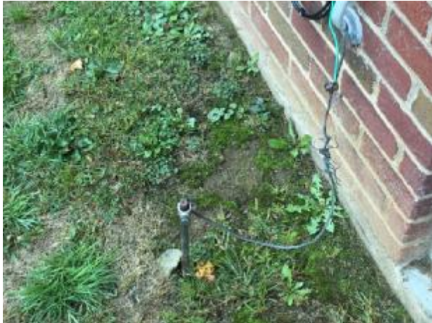
Exposed ground rod
