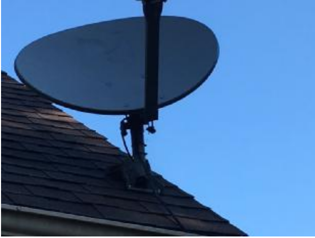
Roof mounted satellite dish.
